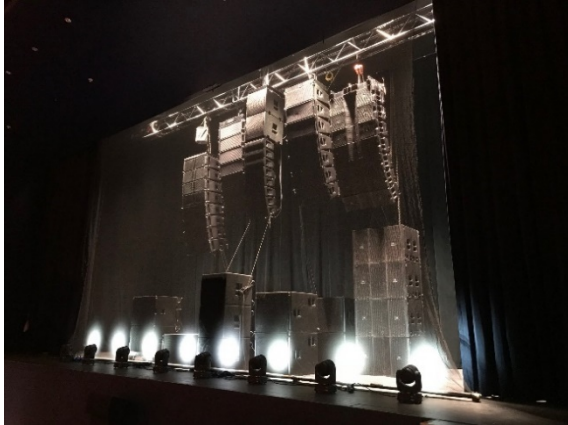
Figure 1. Five systems installed. The main arrays suspended from a truss, subwoofers on the stage.
