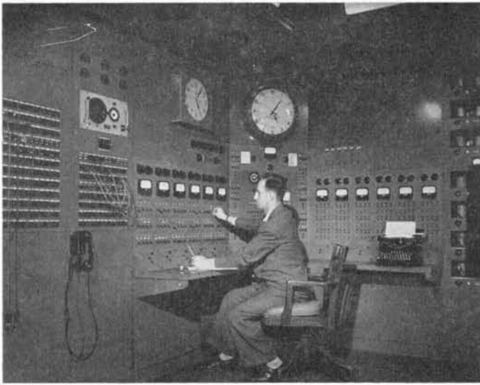
Fig. 1. An installation of twelve standard volume indicators, on an equal number of outgoing program circuits in the CBS shortwave master control room.
