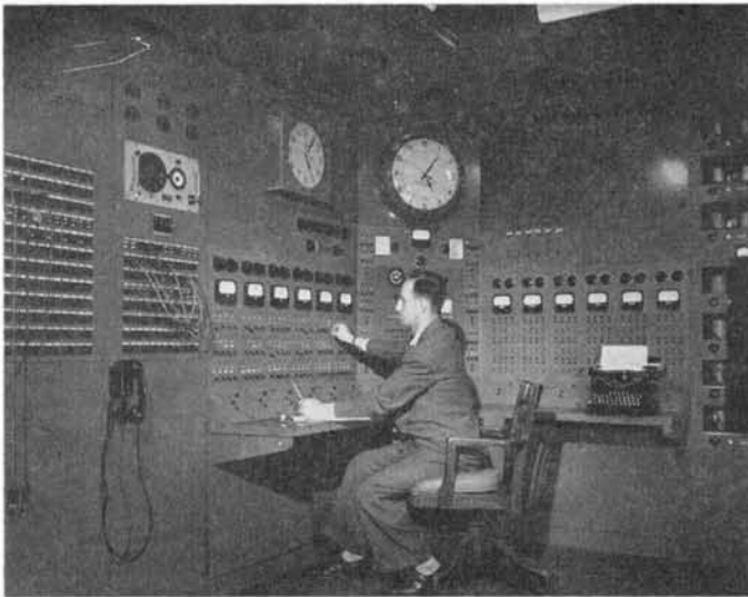
Fig. 1. An installation of twelve standard volume indicators, on an equal number of outgoing program circuits in the CBS shortwave master control room.
